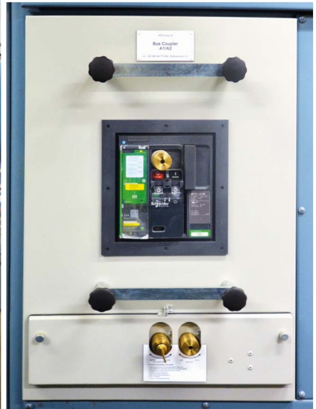
An EDS retrofit low voltage air circuit breaker replacing the Ottermill type OMA24 bus-section.
