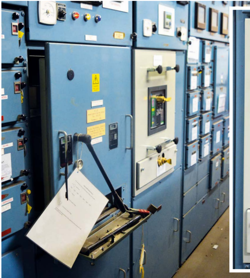
The original Ottermill low voltage air circuit breaker in its withdrawn position (left), and an EDS retrofit such circuit breaker (right).
